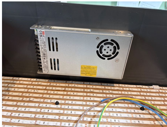
The Mean Well LRS-350 12v 350W transformer mounted inside the Euro Container
