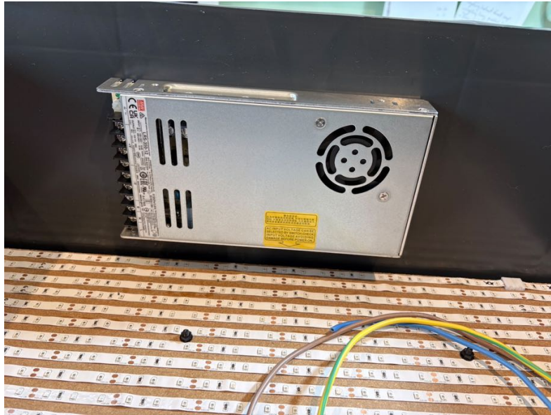
Transformer positioned on the side of the box
